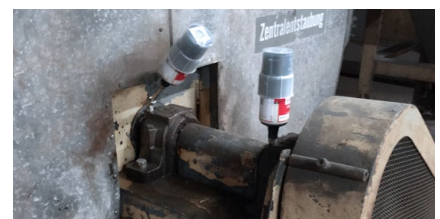
Bearing lubrication on Blowers & fans
