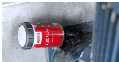
Bearing lubrication on a pump
