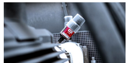
Bearing lubrication on Blowers & fans
